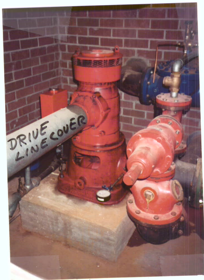
Well \frac{1}{2} Pump
