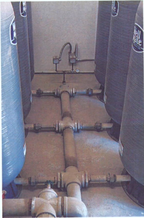
Inside well house
