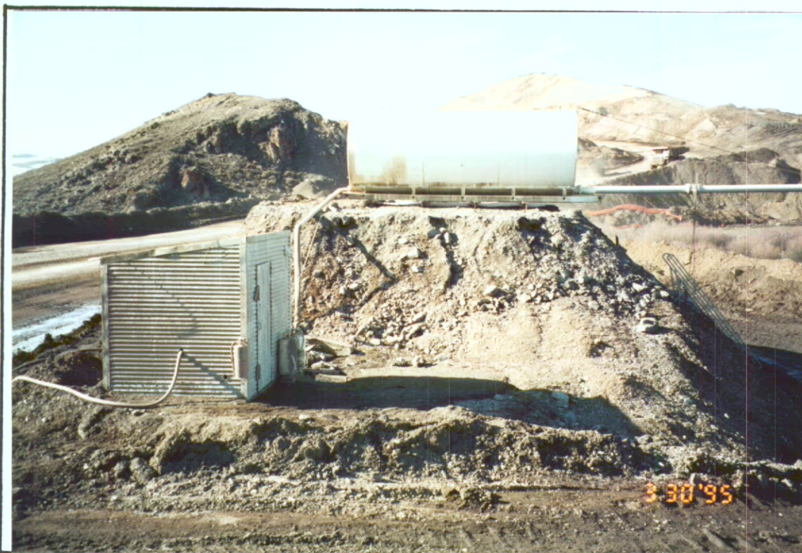
WATER STORAGE TANK AND WELL HOUSE POINT OF DIVERSION
