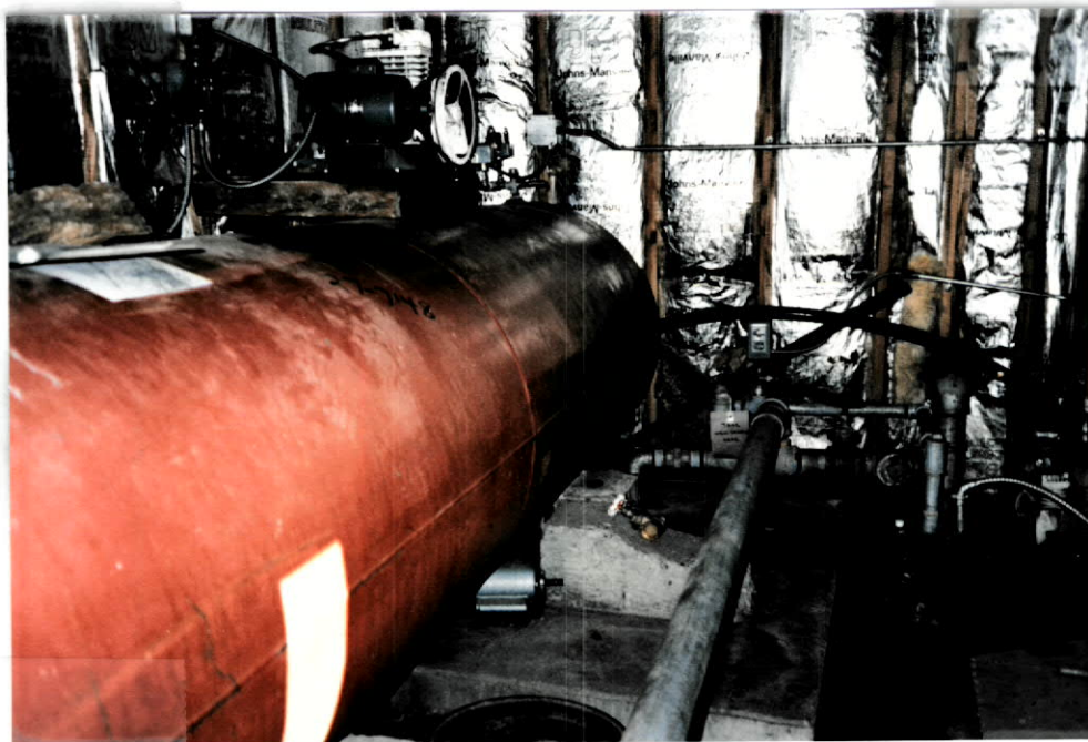
well & Pressure tank inside well House
