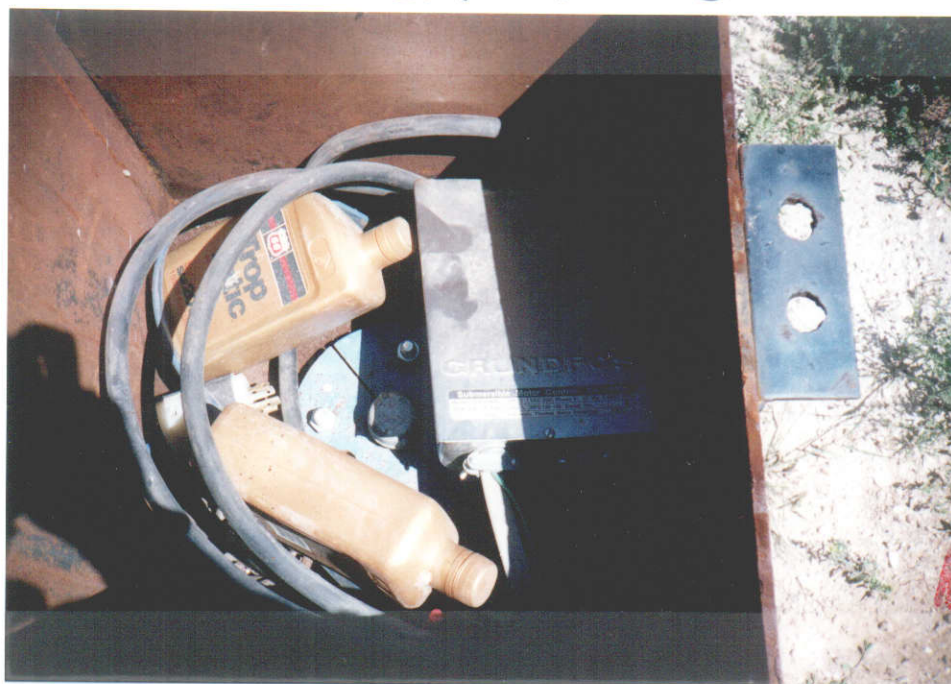
INSIDE OF BOX ON WELL CASING
