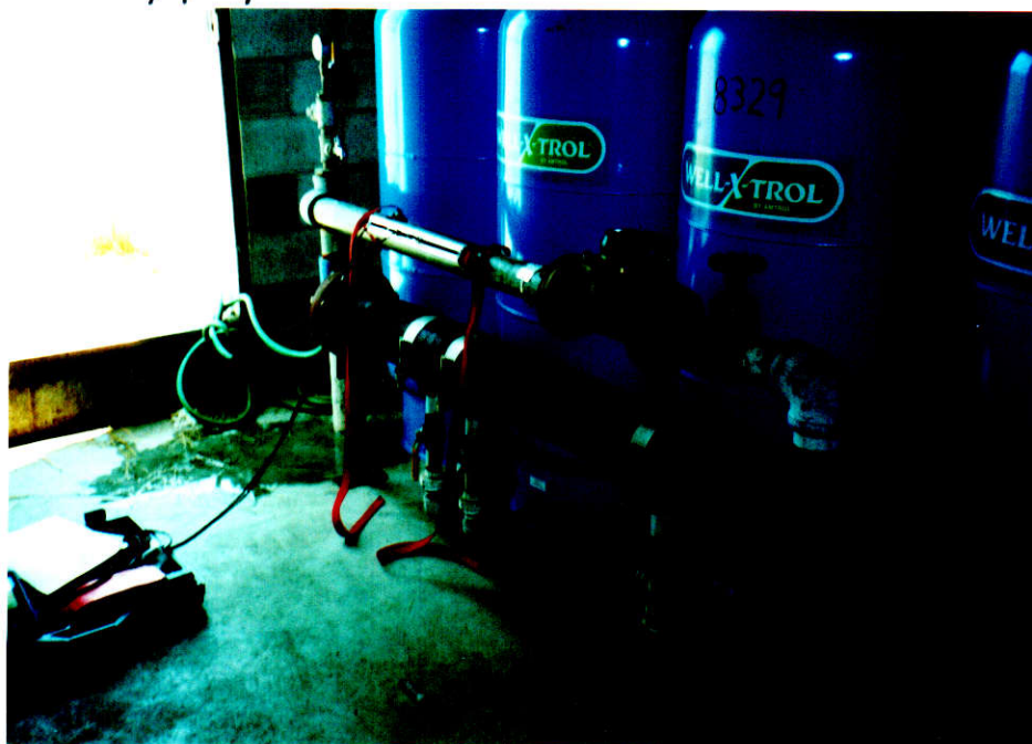
10 hp pump measurement
