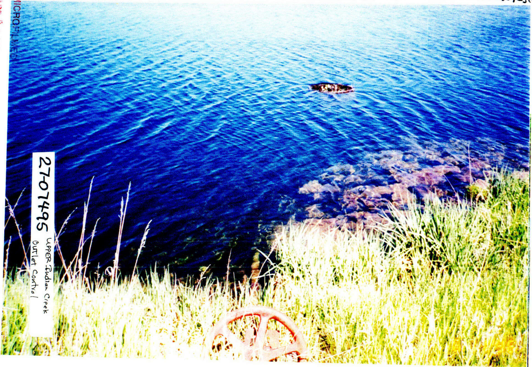
Outlet Control Upper Indian Creek Reservoir
