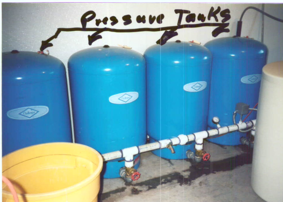
looking east at Pressure tank (4)
