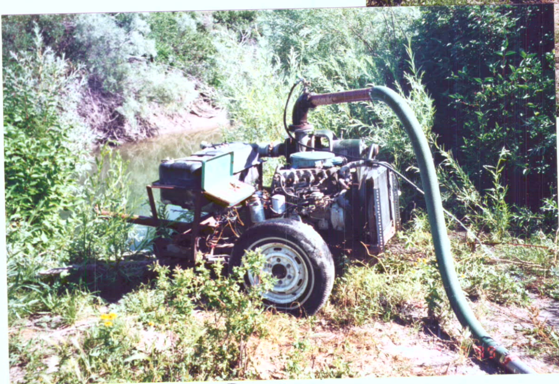
DIVERSION PUMP & MOTOR
