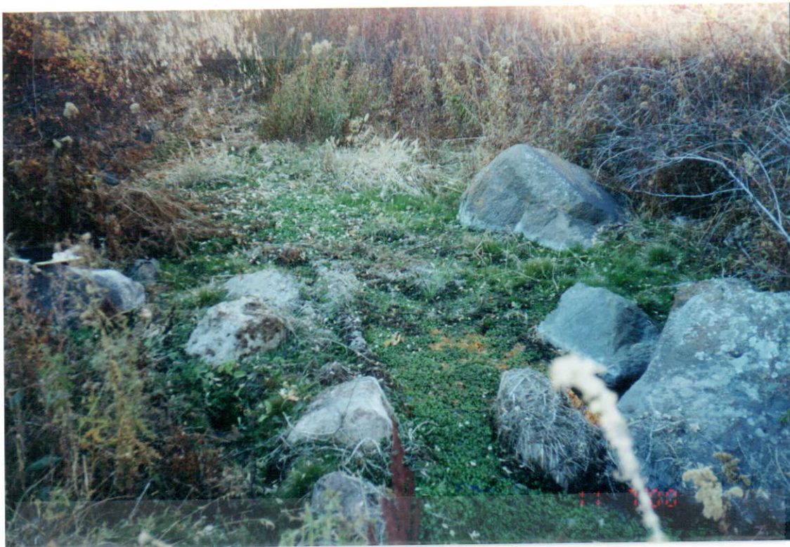
Seepage Below Upper Diversion (Pipeline In Photo Center)
