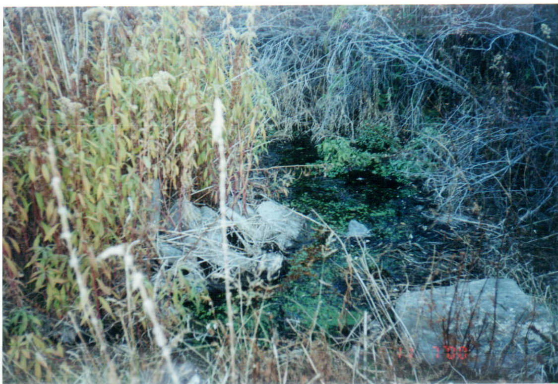
Seepage From Pipeline Below Diversion
