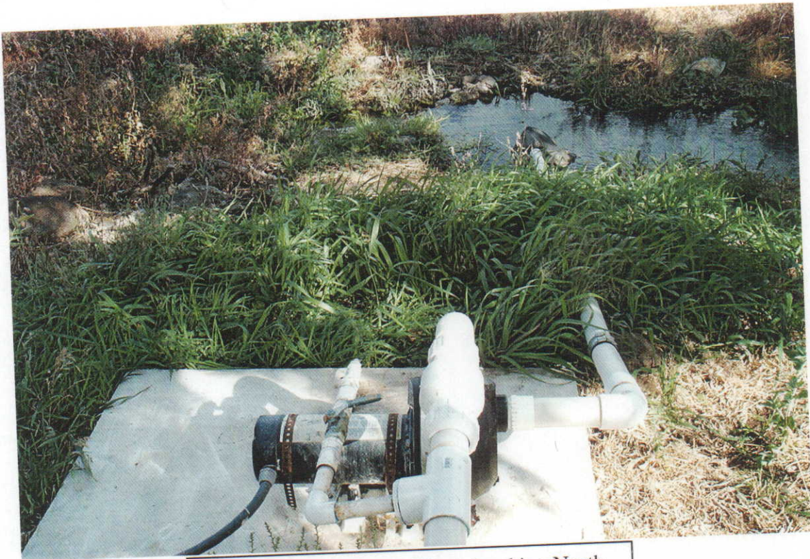
McLeroy Pump In Side Ditch Looking North By J E Stanton 9-9-03 App 47-17100
