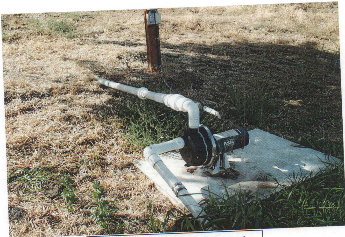
Pump & Mainline Looking Southwesterly By J E Stanton 9-9-03 App 47-17100
