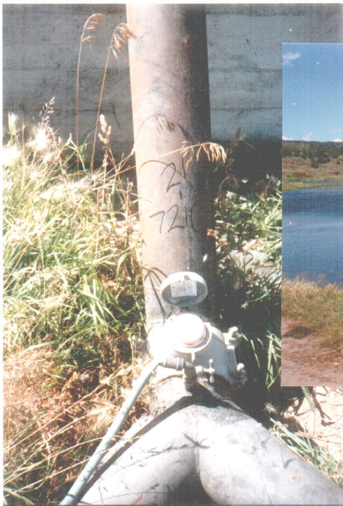
REDIVERSION PUMP FLOW METER
