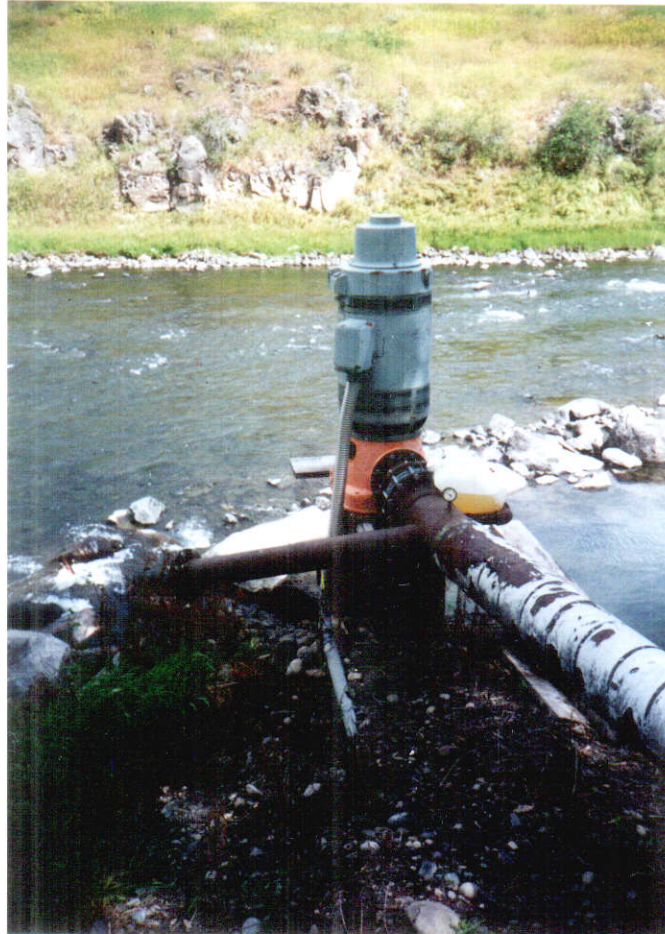
Plate 1 - Pumping station at point of diversion.
