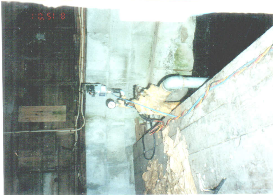
Inside pump house
