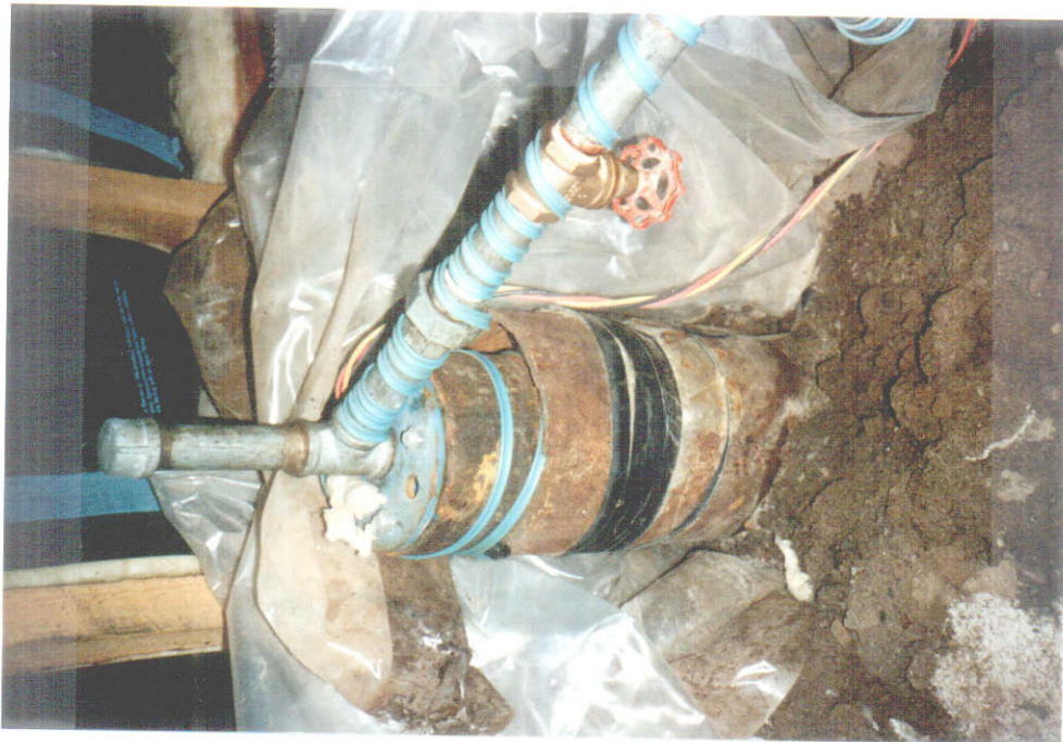
WELL CASING SHOWING LEAK FOR SEAL.
