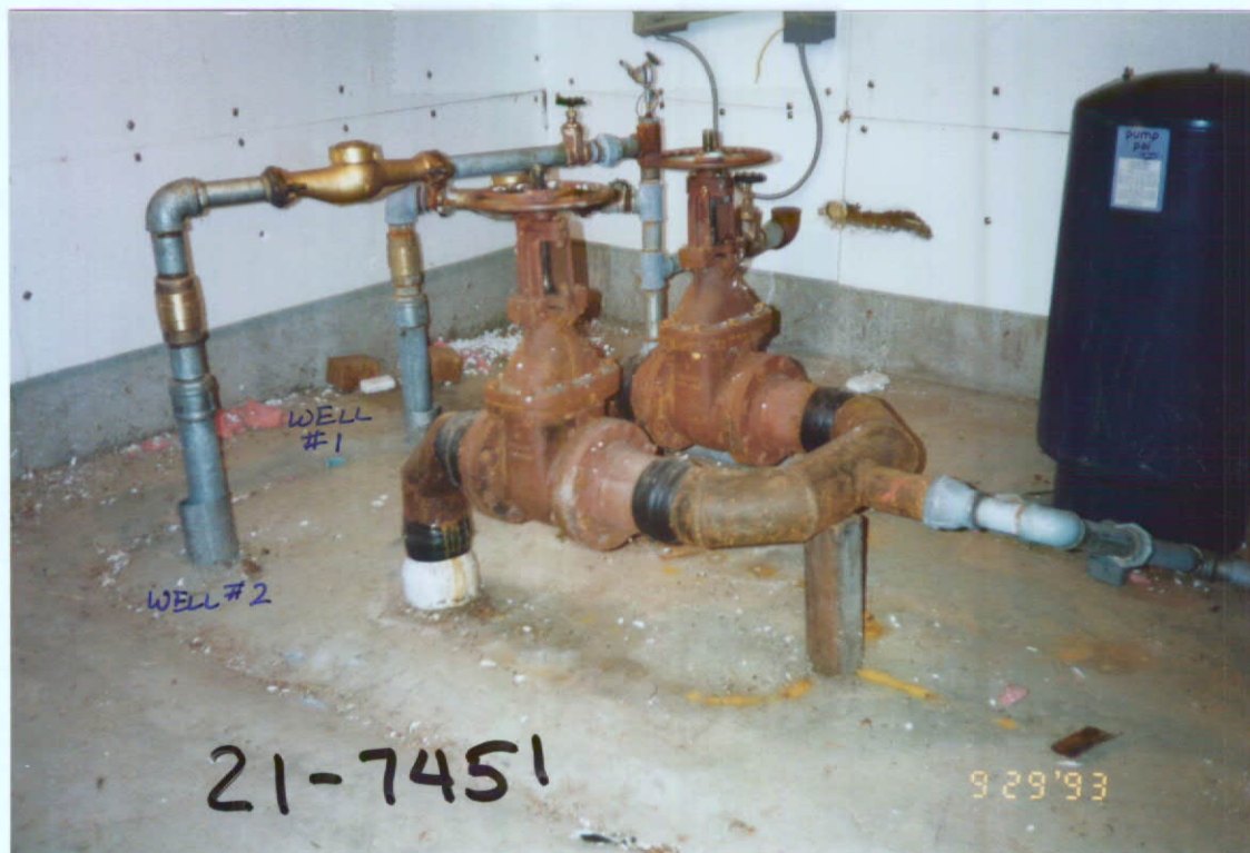
VIEW OF INSIDE PUMP HOUSE
