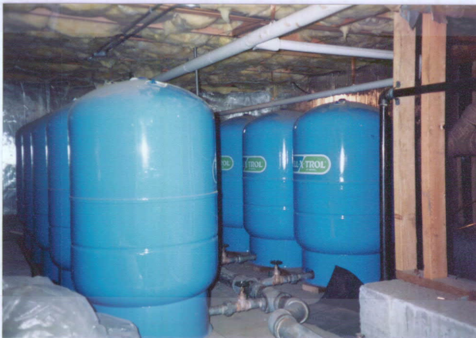
Fig. 3 - Pressure tanks in crawlspace beneath lodge.
