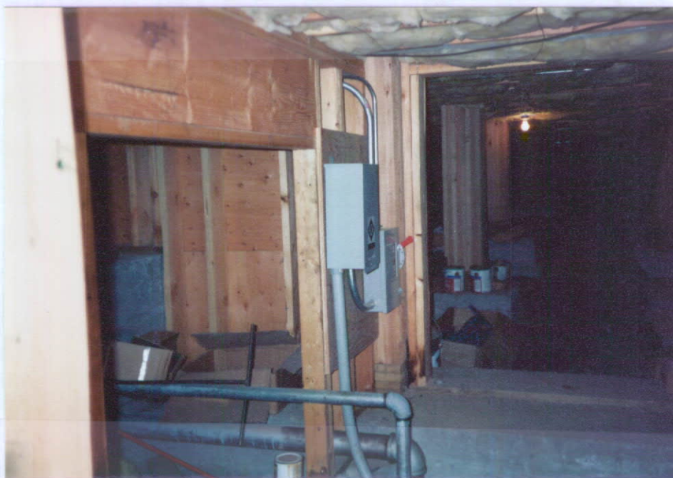
Fig. 4 - Control boxes inside crawlspace beneath lodge.
