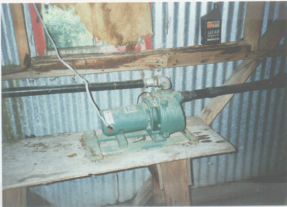
Fig. 3 - Centrifugal pump located inside pumphouse.
