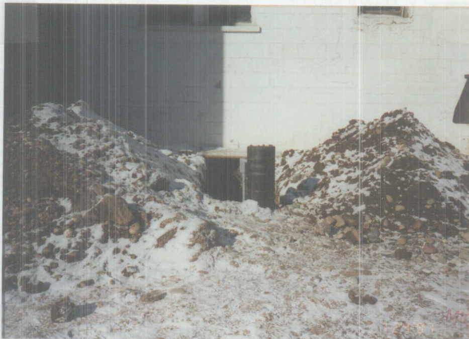
New well in front of plant
