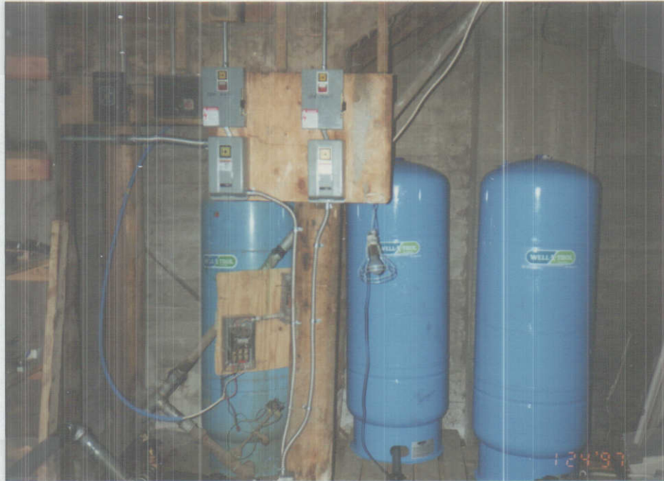
Original well system in Basement of Plant
