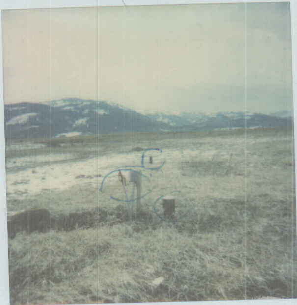
Pump power and wells # 3 and 4
