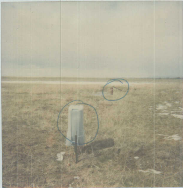
Well # 2 and Power under plastic cover
