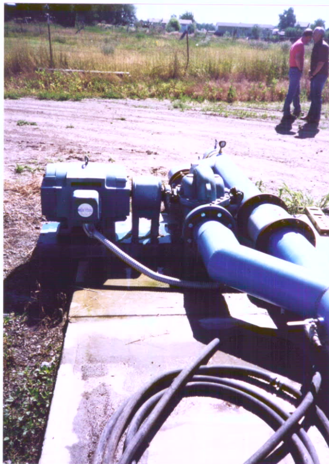
Plate 3 - Closeup of booster at point of diversion.
