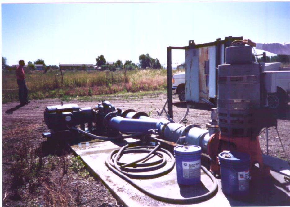
Plate 2 - Complete system at point of diversion. View looking east by southeast.
