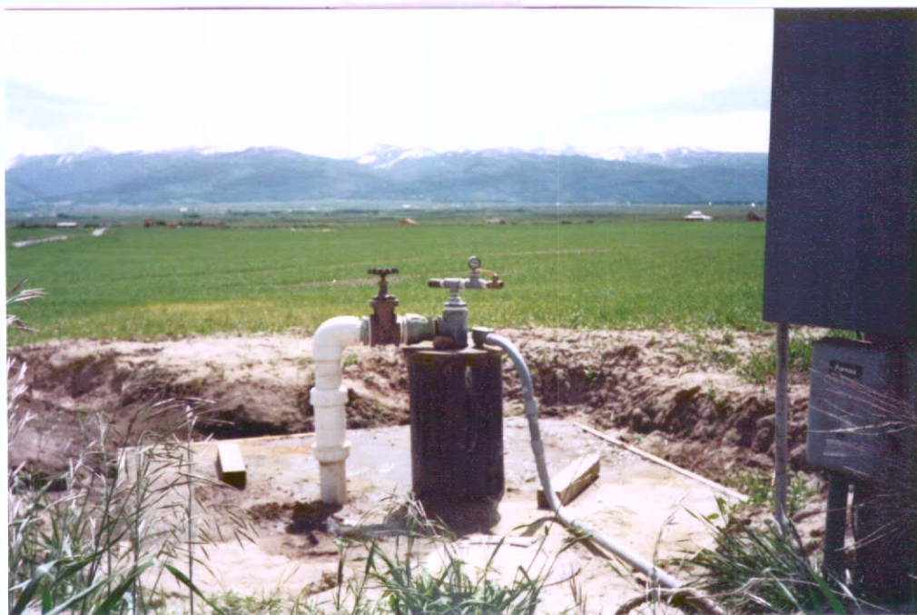
well with 30hp subm. pump, (Locking East) 18" casing
