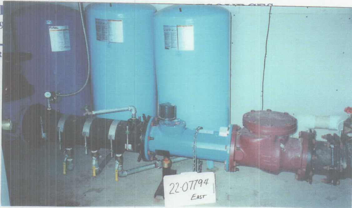
Control Valves, Pressure Tanks, Flow Meter East Well House
