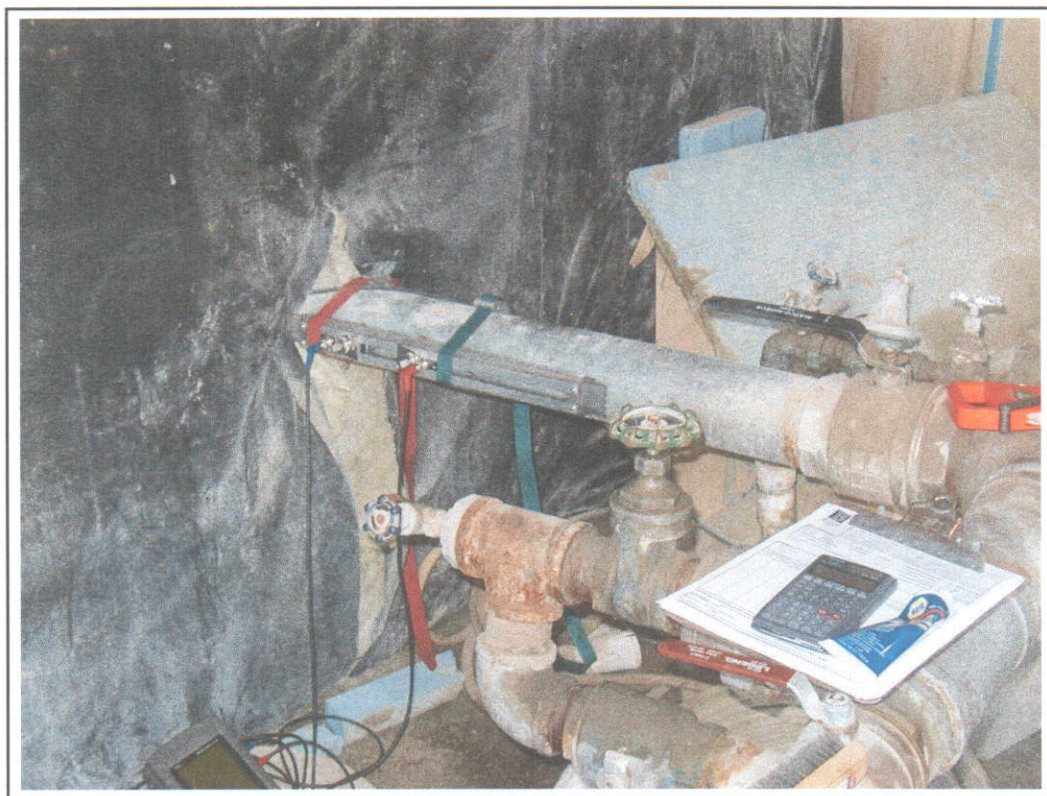
Pipe to irrigation with flow meter attached
