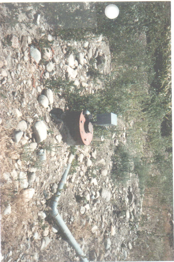
Submersible well & motor & pump.
