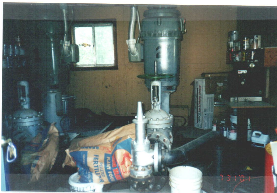
Re-lif Pumps For Snow Making (Looking East)
