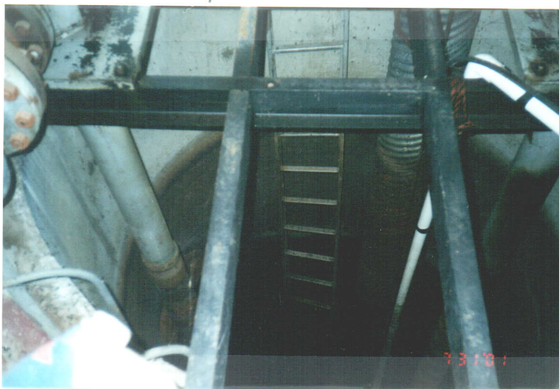
Sump With Pump Intakes
