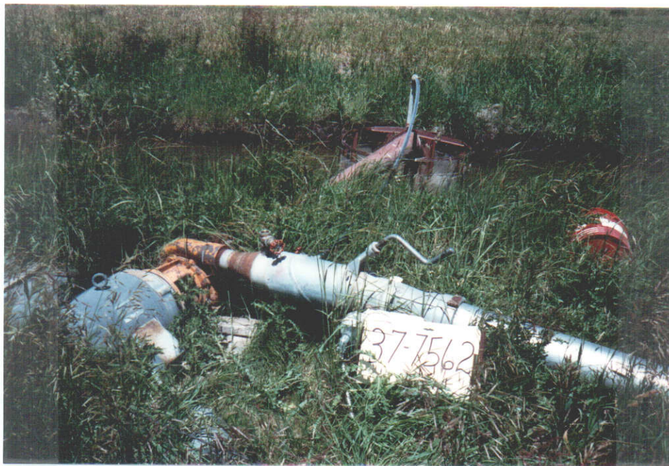
Pump in Upper Ditch to Sprinklers
