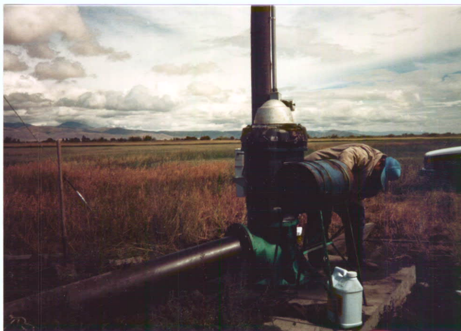
well motor & pump.
