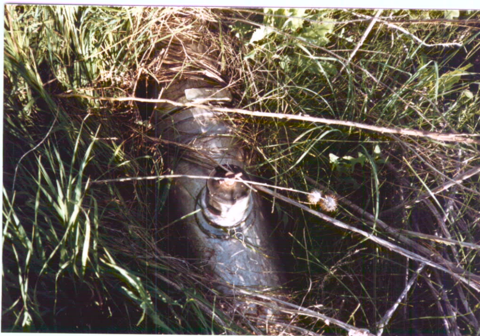
5" Riser For Discharge Into Canal ditch
