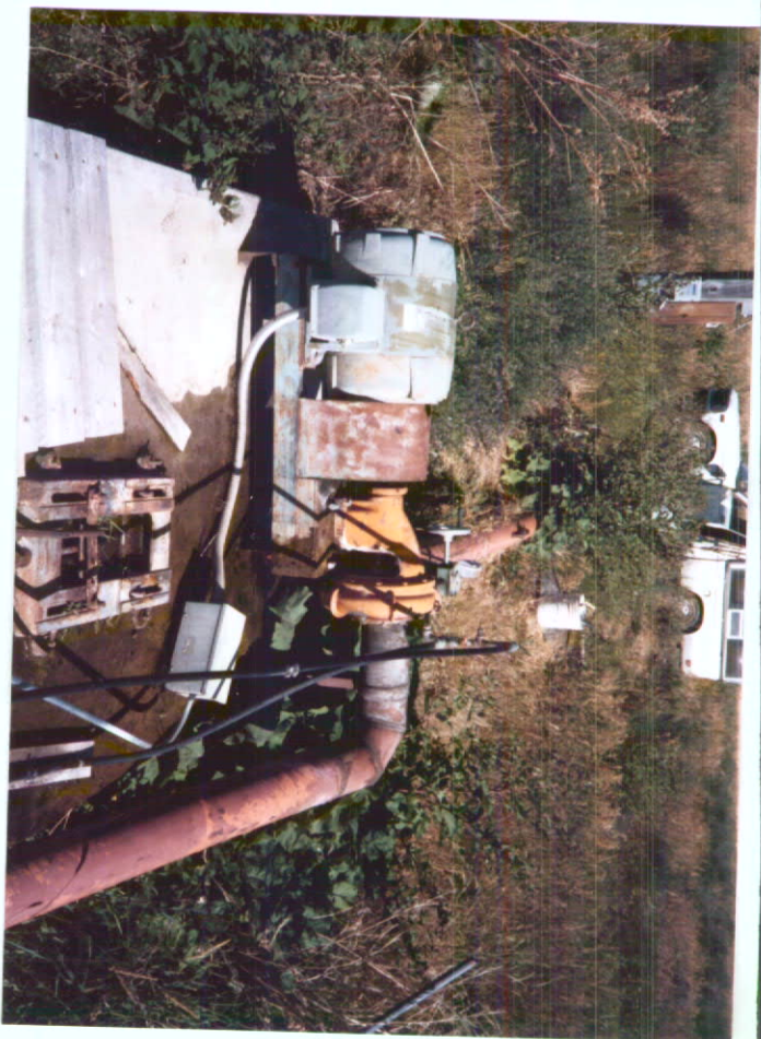
Motor & pump @ Louder Reservoir.
