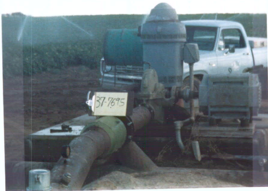
Point of diversion: Access port and flow meter are located on bottom near left hand corner
