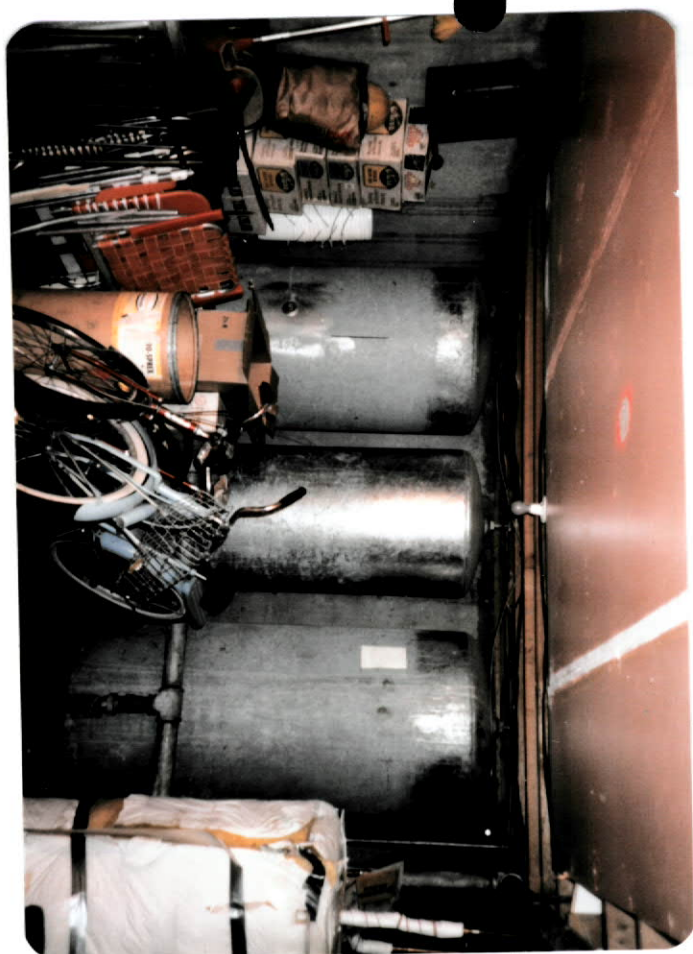
← 3 pressure tanks w/2 1/2" dia inlet and outlet.
