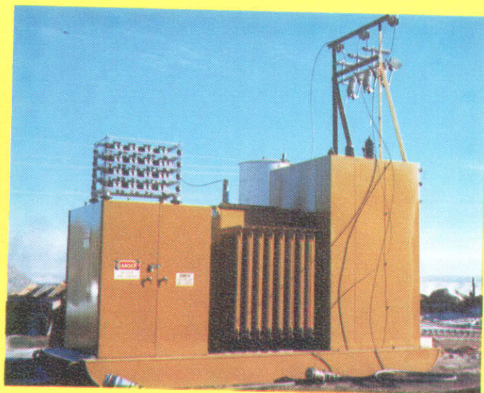
24.9 KV to 5 KV
