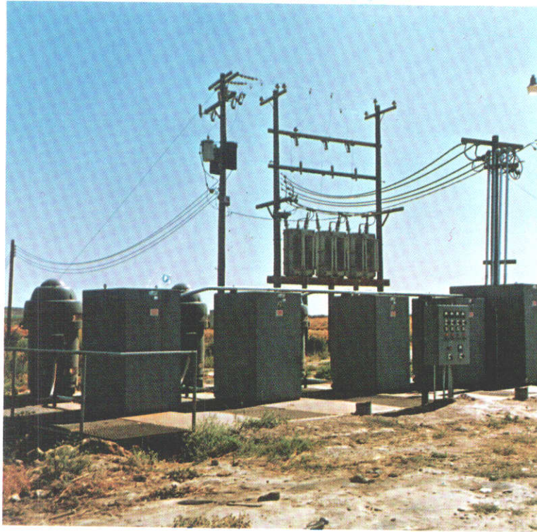
Four 600 H.P. 2300 V. Panels and One 1200 Amp. Air Breaker Panel
