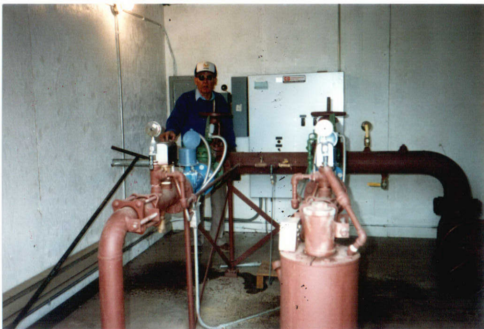
Inside Well house #2 ↑ Well Inlet of #1 Well
