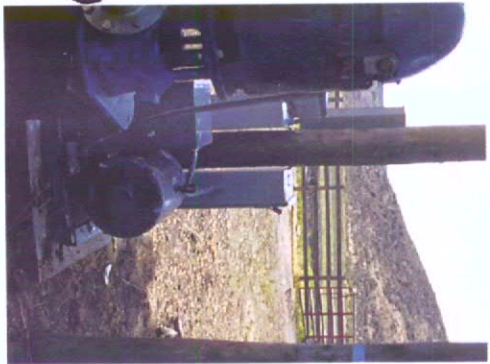
Well, Booster Pump, and GPS Tag A0004195
