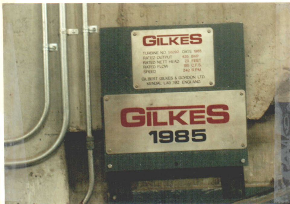
Photos of the smaller generator Permit No. 37-7943
