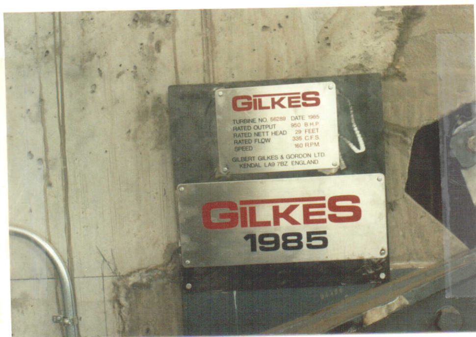
Photos of the larger generator Permit No. 37-7943
