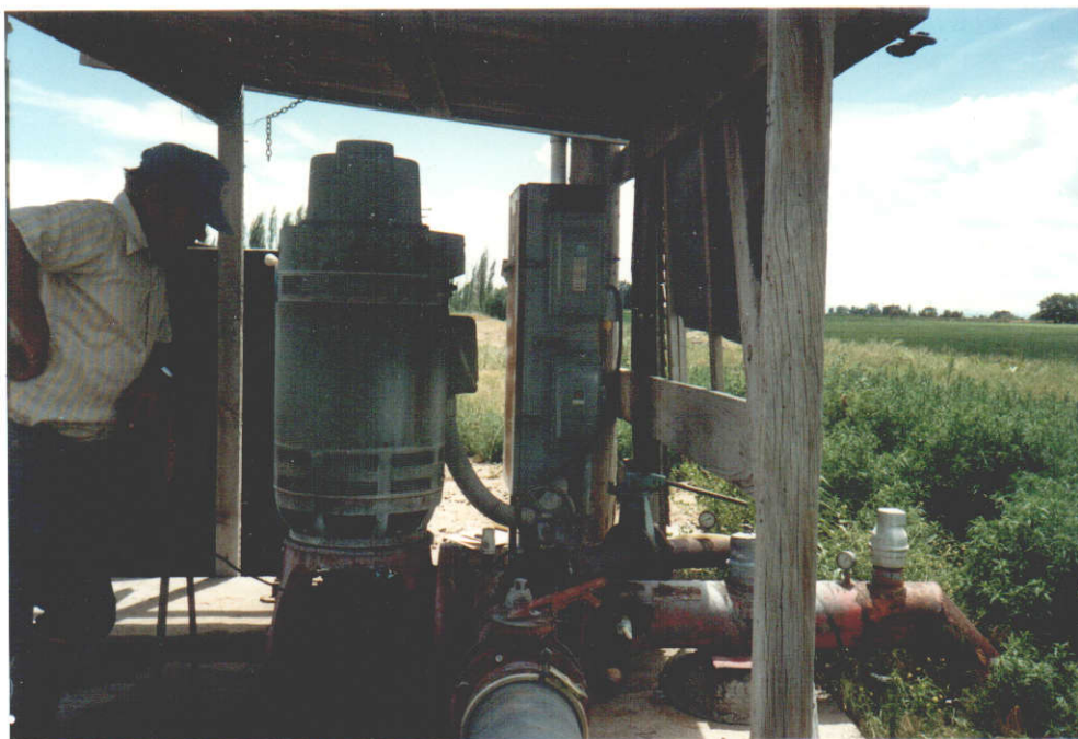
150 HP Turbine Pump and 3 Lines,
