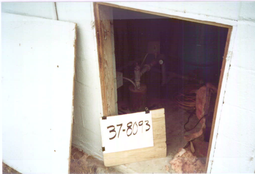
main well Point of diversion and pressure tank
