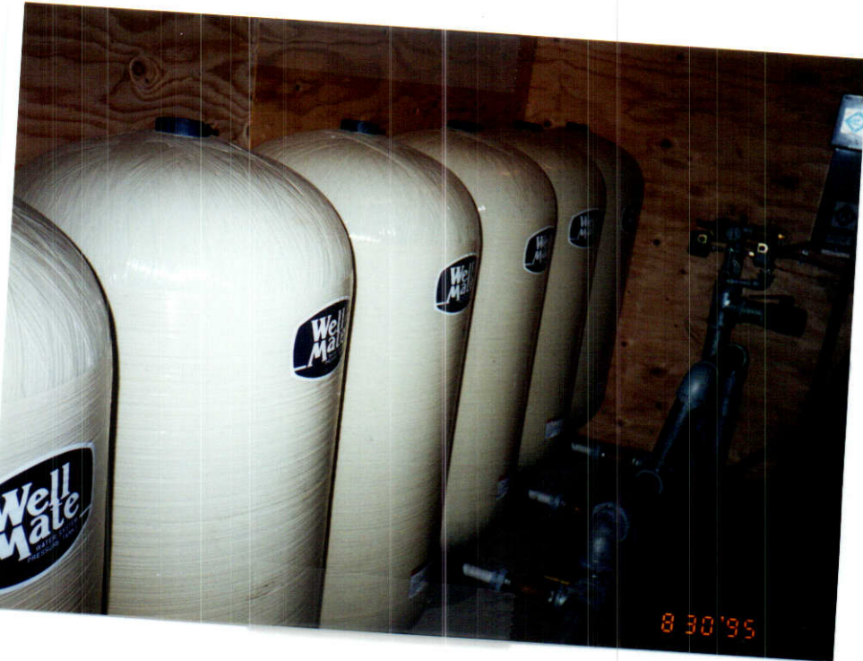
P.O.D Pressure Tanks
