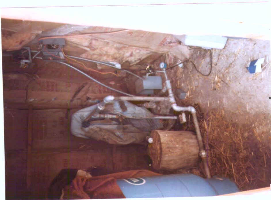
P/O - well & P. tank
