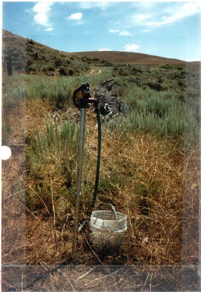
Frost Free Hydrant. at Cabin
