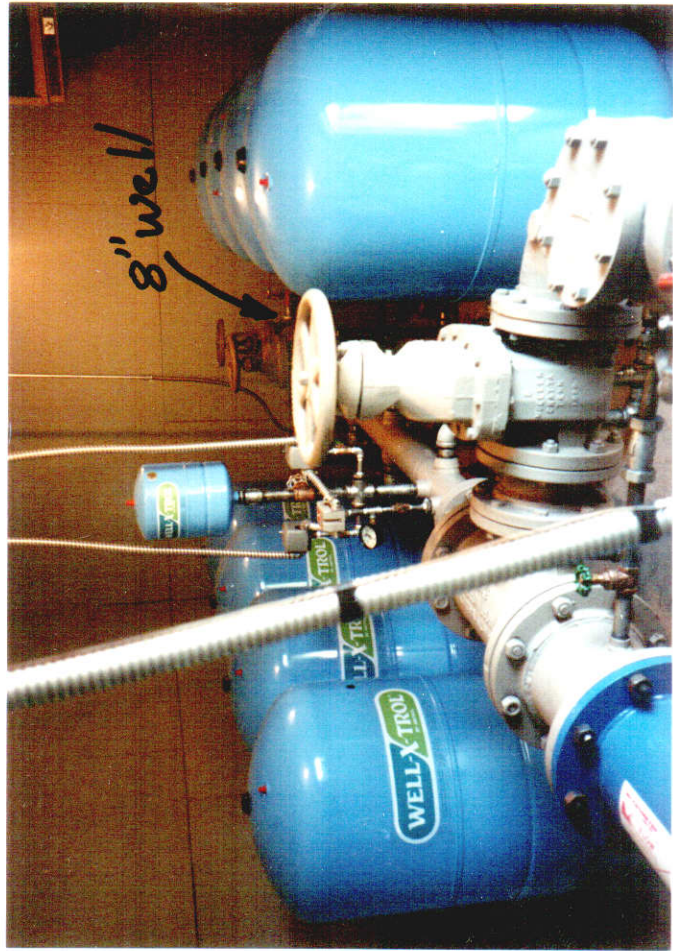
Pressure Tanks in Well house
