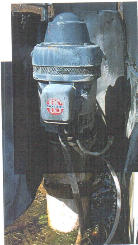
50hp Berkeley Pump A0007943
