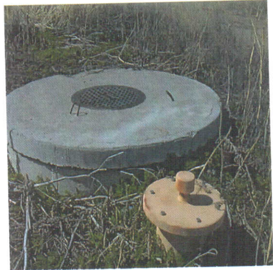
Submerged 25hp STA-RITE Pump, A0007942
