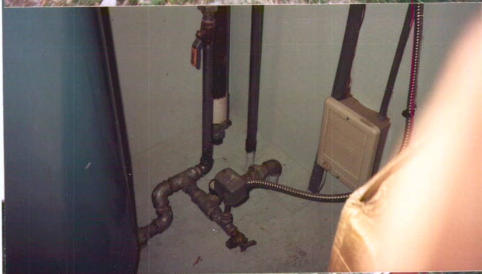
30 gal Pressure Tank
