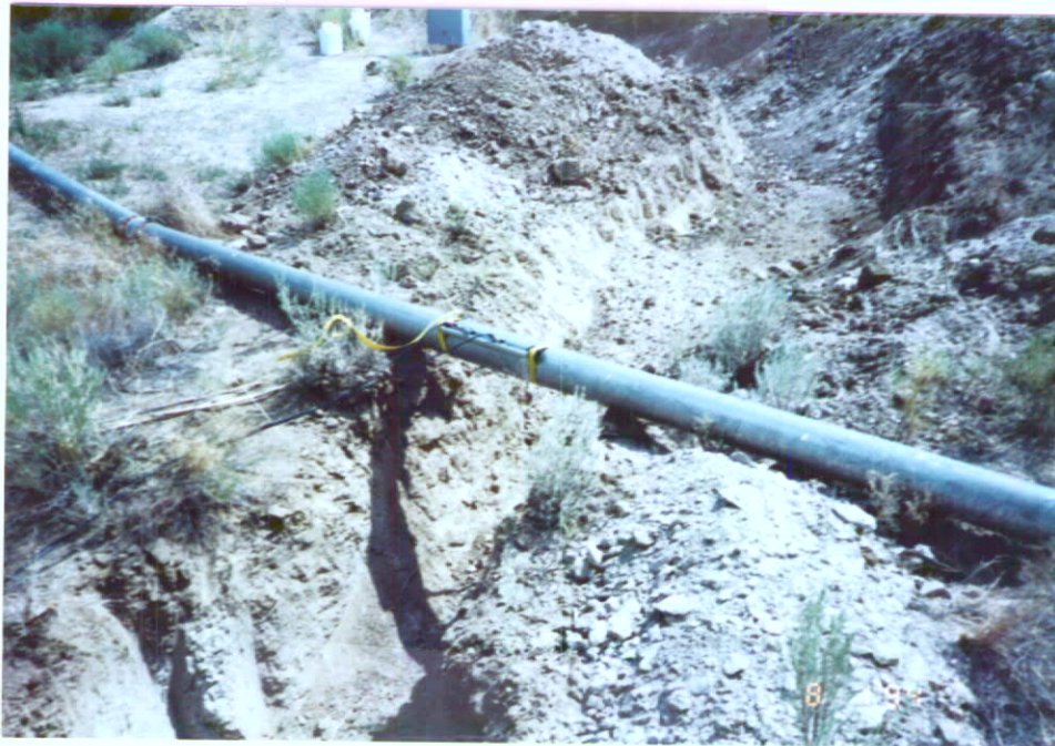
#3 Polysonic installed on line going to pivot.
