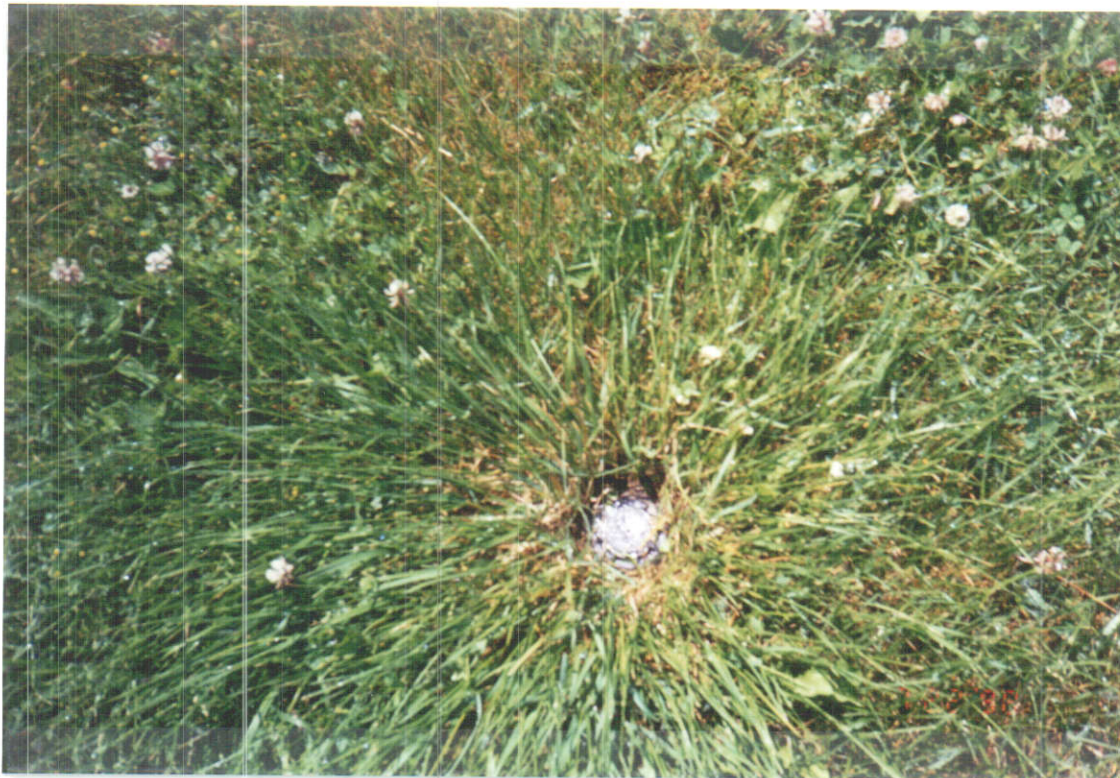
Buried Pop-Up Sprinkler Head
