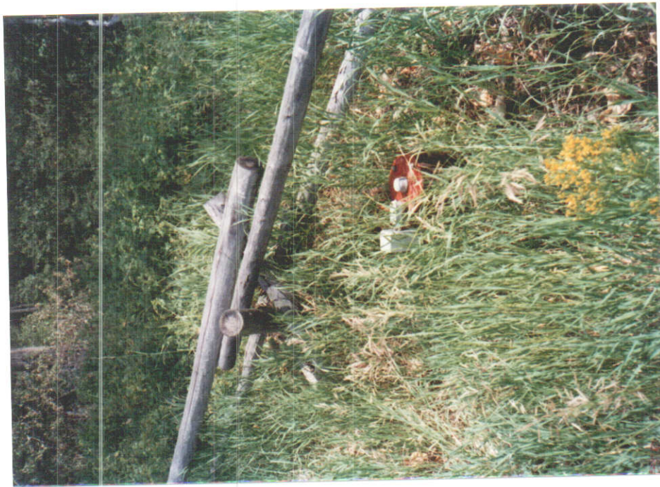
8" well P/U submers. pump
