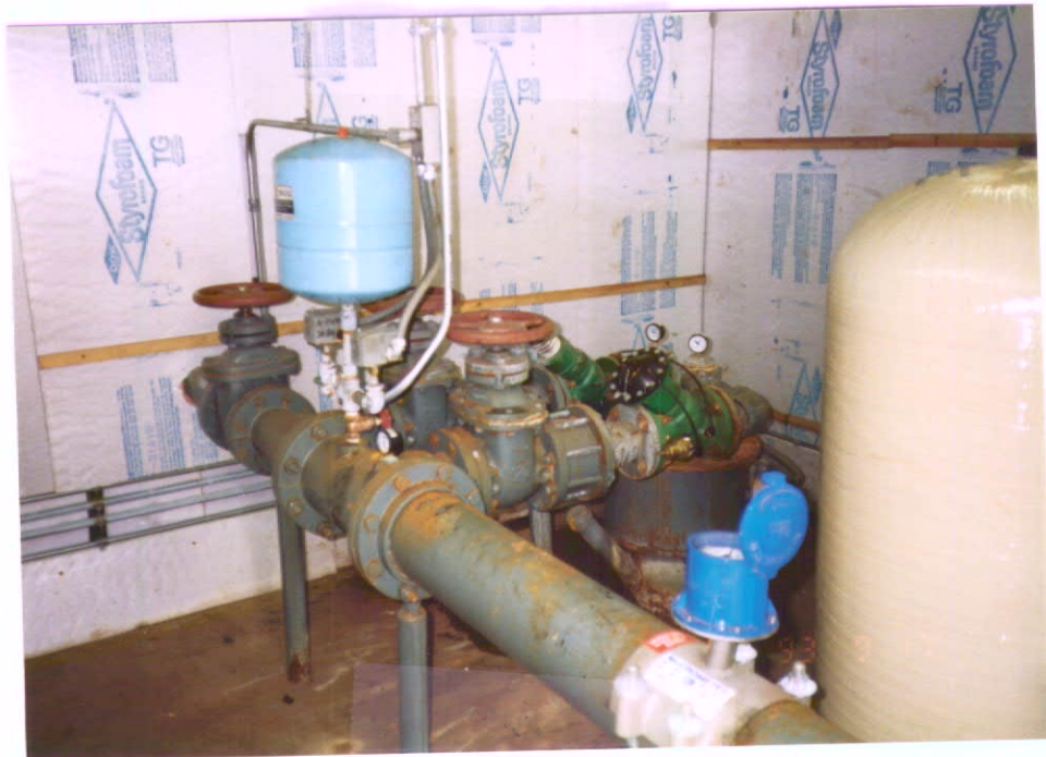
#1 PIR located in well house.
