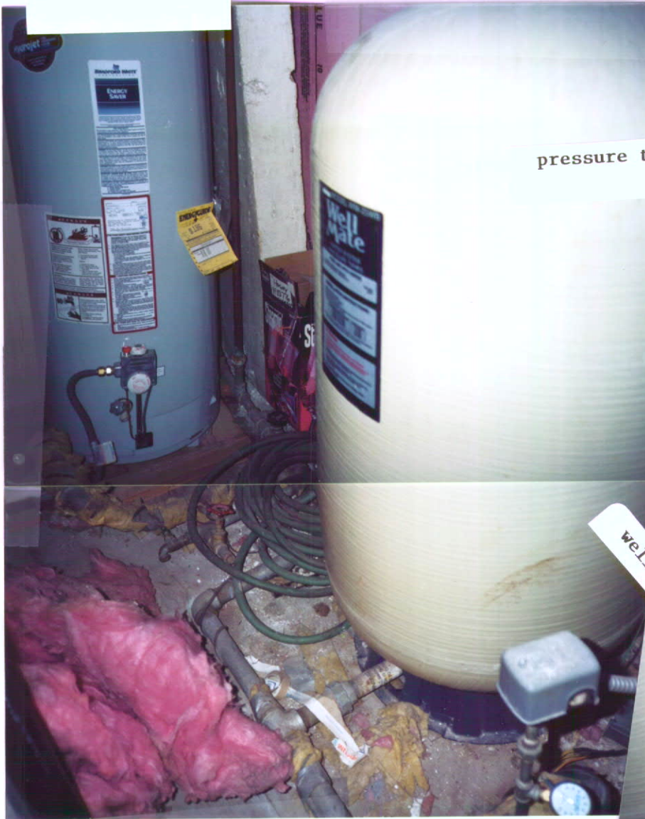
hot water tank
