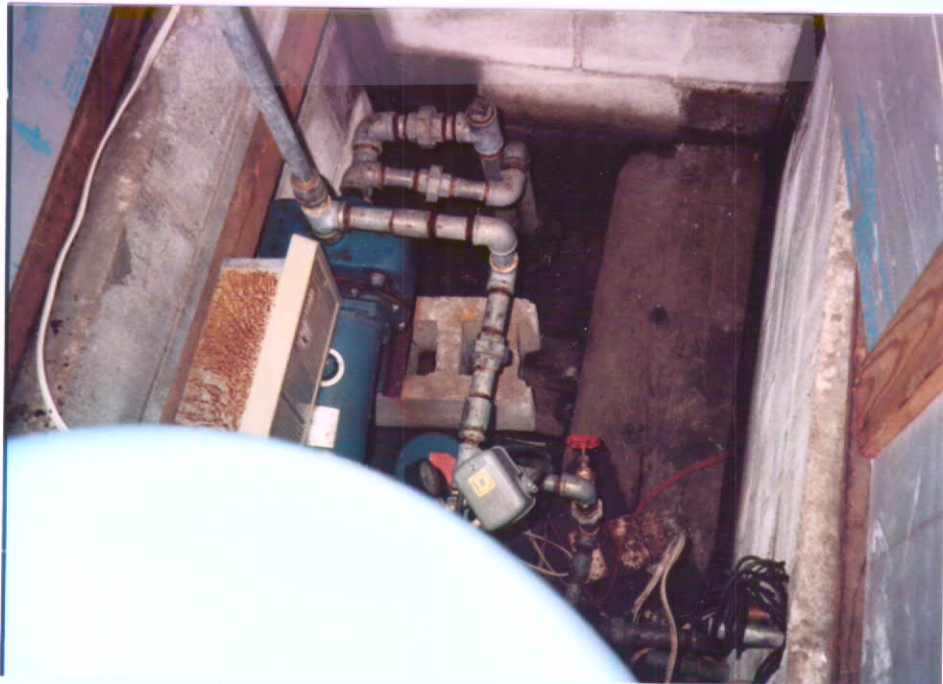
P/D #3 - back up, fire protection
