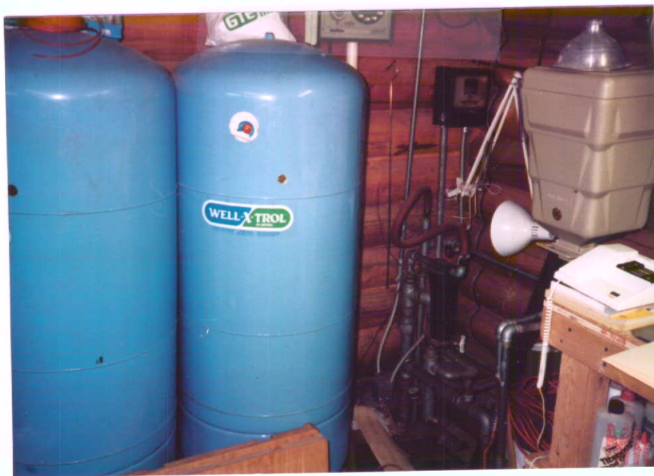
tanks, piping for well #1
