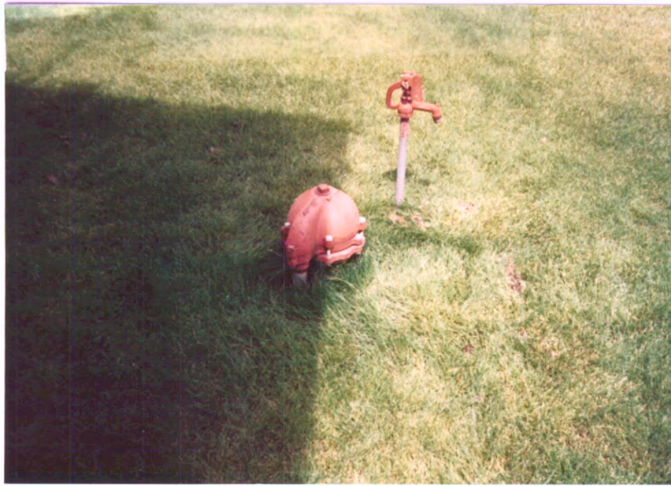
P/D #1 - main well for irrigation and domestic uses
